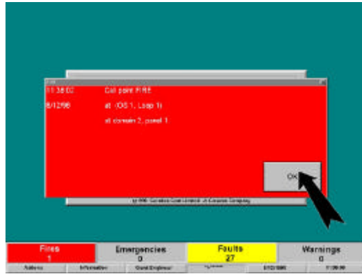
Figure 31-1 Display showing report of fire jnpic3
