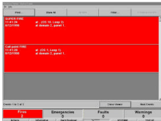
Figure 31-3 Fire event log showing current fire events jnpic4
